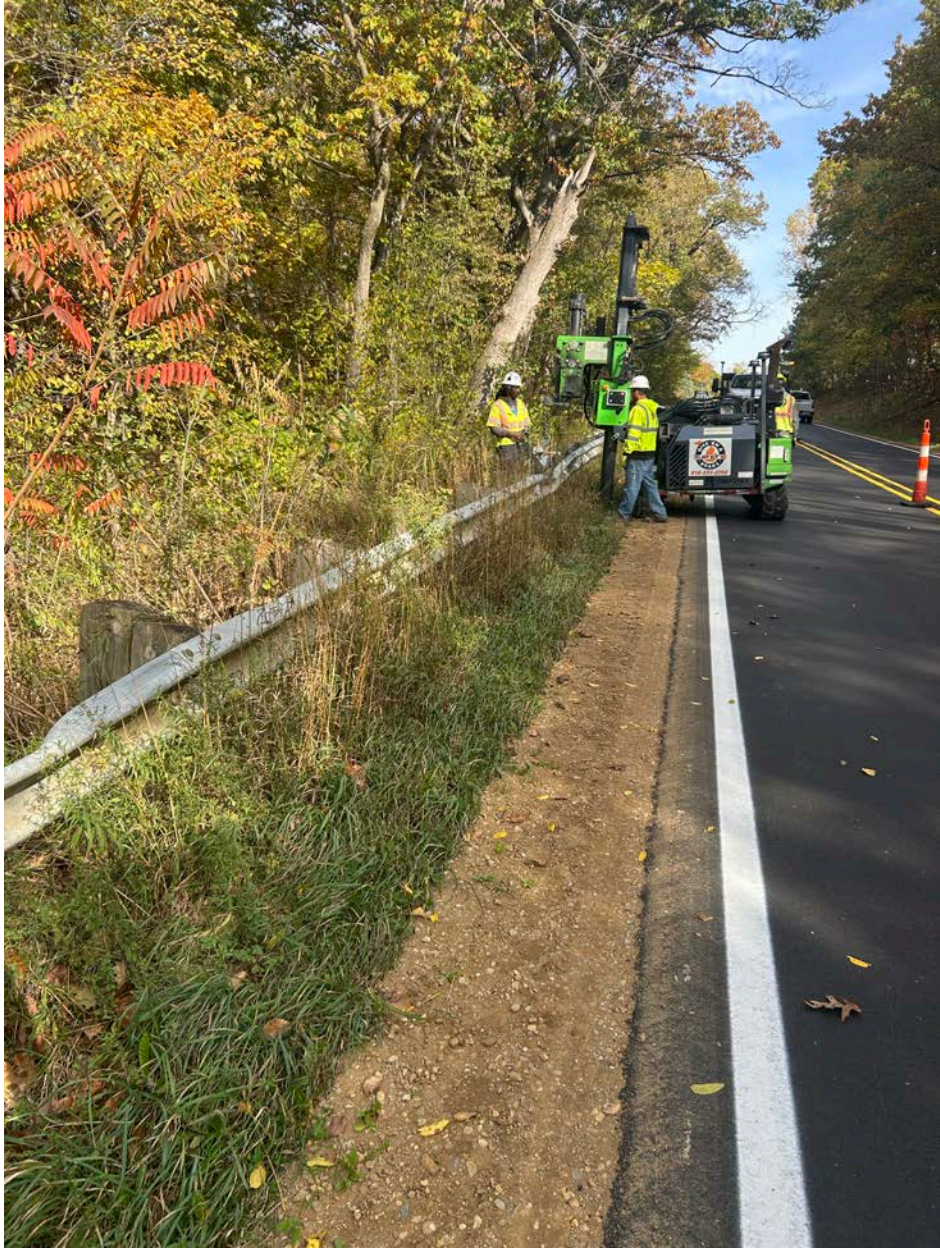
Guardrail Adjustments on Moscow Road in between Farwell Lake Road and Buckman Road.
