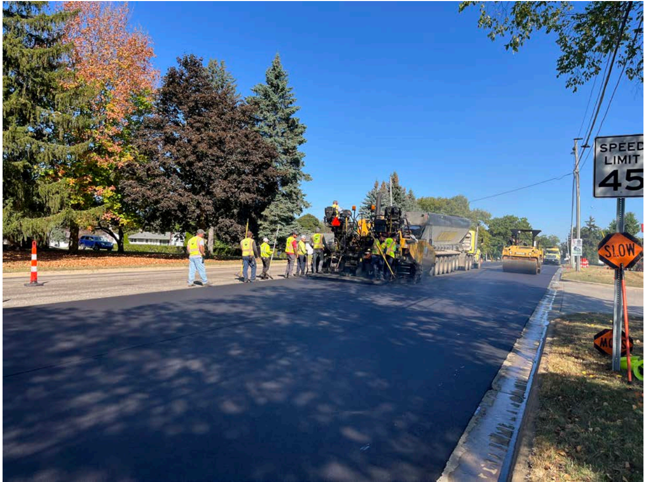
Lakeland Asphalt Top course paving at Lansing Avenue and Parnall Road intersection.
